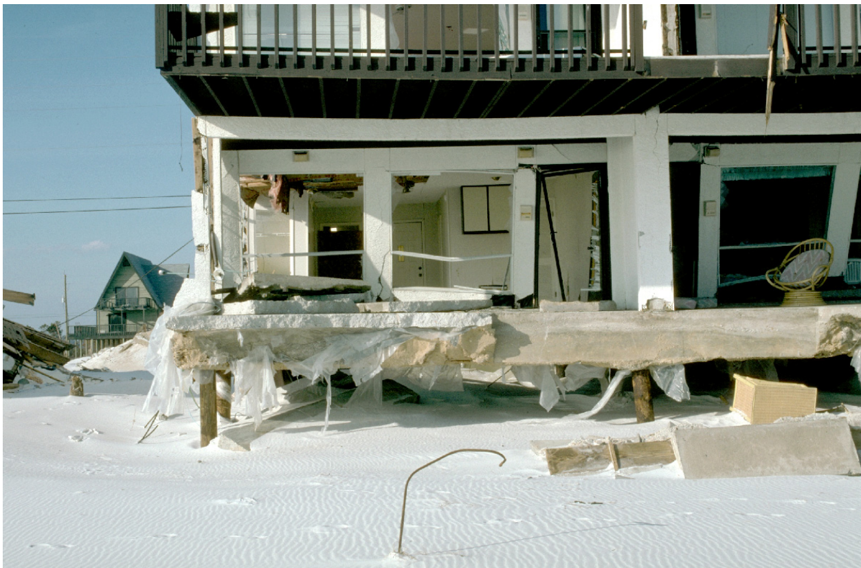
Figure IV-1-14. Hurricane Opal damage at Navarre Beach, Florida, November 1995. The sand underneath the concrete slab washed away, and the unsupported floors collapsed
